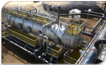
Onshore Deoiling Water Treatment
