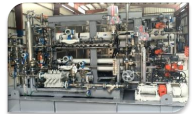
Offshore Ultrapure Water Generation Package
